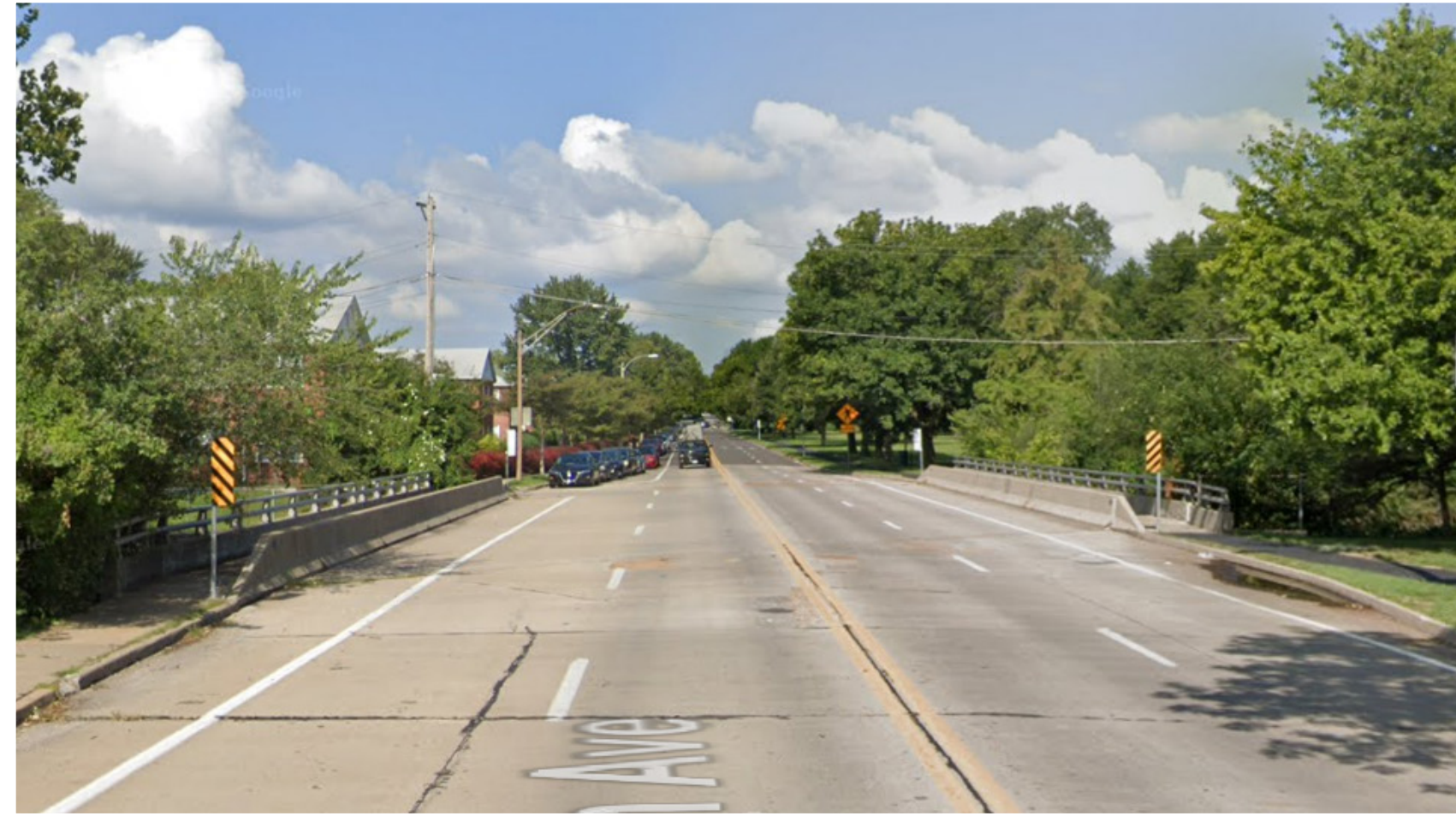
EXISTING CONDITIONS Looking West from Vernon Ave. & River Des Peres bridge crossing
