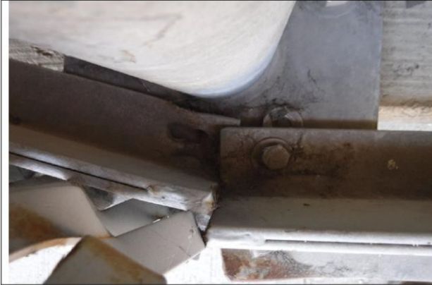
Photo 37 : Damaged Fence – Light Structure see page 8
